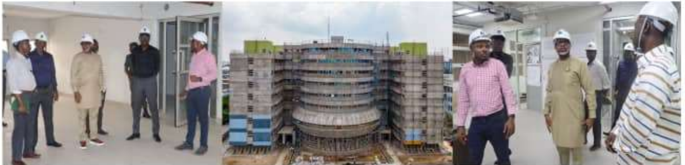
MD, LASAA, Prince Adedamola Docemo and management team during an inspection to the Agency's new office complex, at the Revenue House, Alausa, Ikeja, currently undergoing renovation
