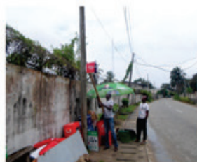
ILLEGAL DEPLOYMENT OF FLAGS AND TIN PLATES (SUCH WILL BE REMOVED AS SEEN IN THE PICTURE ABOVE)
